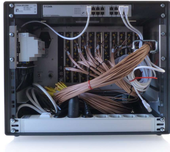
Rear View, with RF cables
